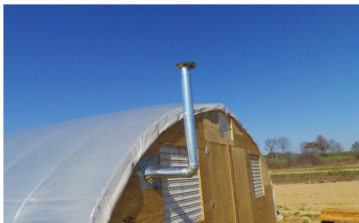
The flue pipe extends over the roof line by several feet and has a cap in place to prevent flue gases from being blown down the pipe into the greenhouse. (Photo by Thomas G. Ford)
