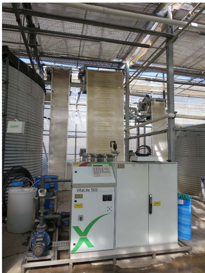
Figure 5. Two-stage filtration. After the storage tank, the nutrient solution passes through two staged of filtration. The filters in this examples are commonly known as “paper filter”. Following filtration is the UV treatment system.
