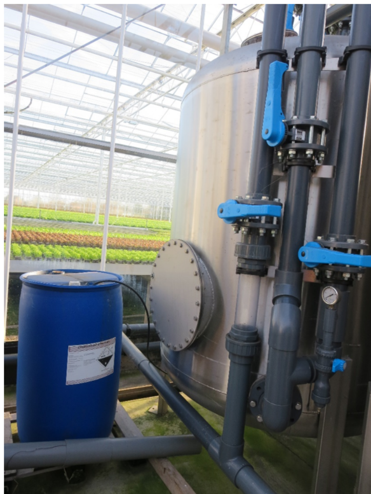
Figure 6. Granular activated carbon (GAC) filter in the metal housing. Next to the filtration system (blue tank) are chelated micronutrients which are injected to replenish the elements removed by the GAC filter.
