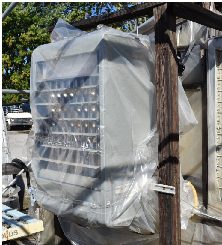
Figure 7. Example of covering a unit heater during the summer months with poly when the greenhouse glazing material was removed. Growers should check the heater for any loose wires or connections or poly that has entered the cabinet. Photo by: W. Garrett Owen, OSU.
