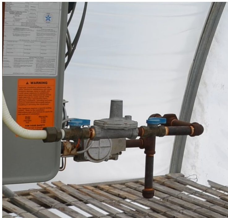
Figure 3. Verify the manual shutoff valve on the fuel line is open. Photo by: W. Garrett Owen, OSU.
