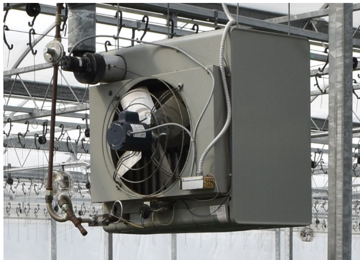
Figure 4. Inspect unit heater electrical wiring and connections to ensure no wires were accidentally pulled loose while the unit sat idle from late spring through fall. Photo by: W. Garrett Owen, OSU.
