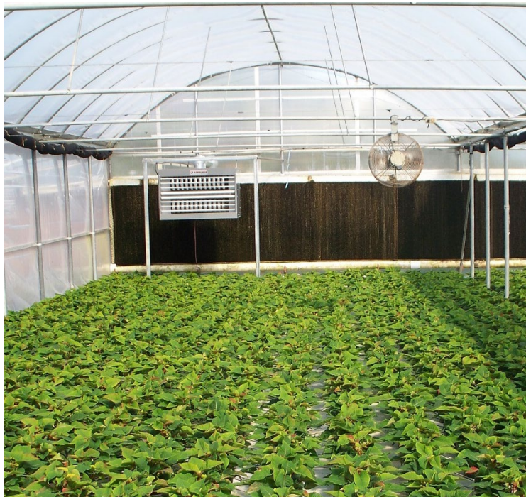
Figure 2. Ensure the unit heater louvers are set so warm discharge air is directed into the production area. Photo by: W. Garrett Owen, OSU.
