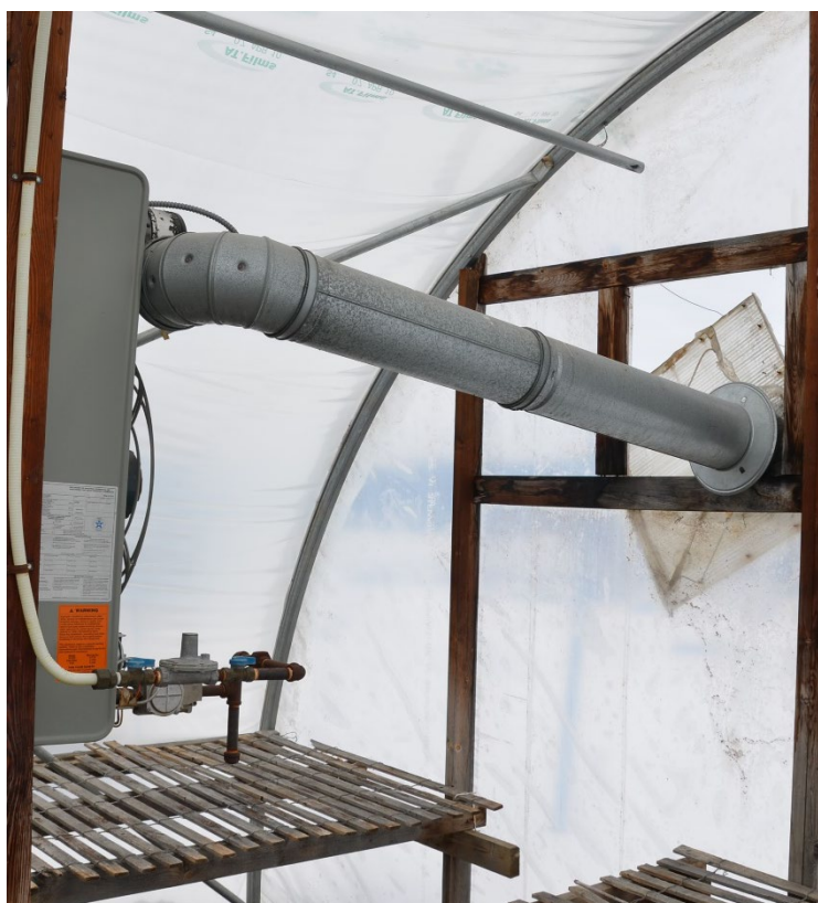
Figure 9. Confirm that the vent stack of the unit heater is securely attached, properly pitched, and terminates outside the greenhouse. Photo by: W. Garrett Owen, OSU.
