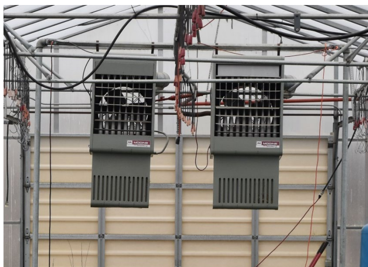
Figure 5. Example of a grower inspecting and cleaning each unit heater burner cabinet to ensure it is free of dust, leaves, insect parts, and plant debris. Photo by: W. Garrett Owen, OSU.
