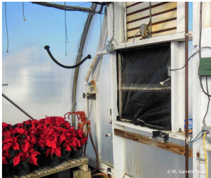
Figure 10. Example where exhaust fans were temporarily covered with plastic sheeting to prevent cold air infiltration prior to an extreme cold weather event. Photo by: W. Garrett Owen, OSU.
