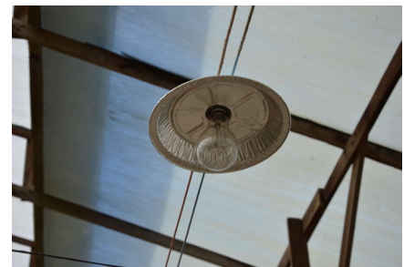
Fig. 4. An incandescent bulb with a reflector pie plate used in greenhouses to provide LDs.
