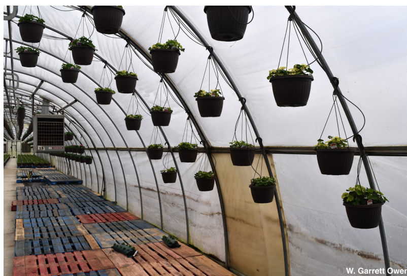
Figure 4. Primary heater mounted 12 feet away from the first bow of suspended geranium baskets.
