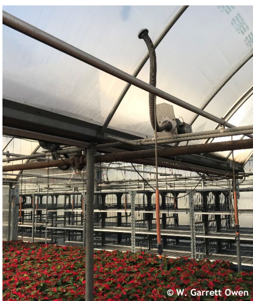
Figure 1. An often-overlooked aspect of greenhouse management is the proper installation of a double-poly inflation system. Photo by: W. Garrett Owen, OSU.
