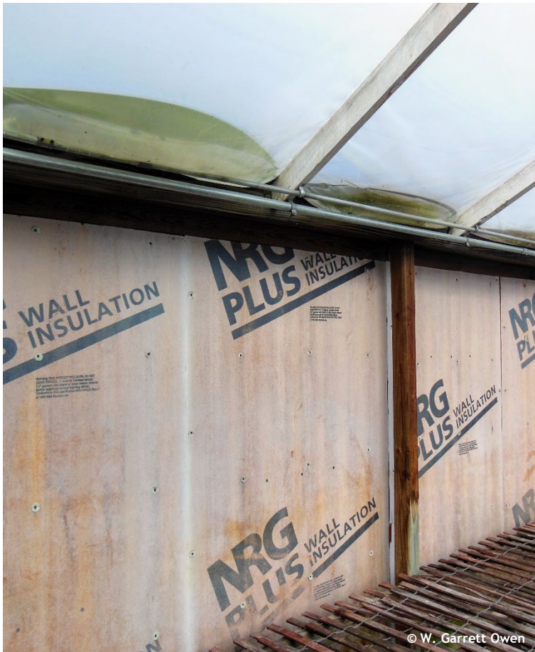
Figure 7. Improper installation of a greenhouse inflation blower fan using humid greenhouse air can cause condensation between double-poly layers, reducing light transmission, accelerating material degradation, and fostering mold growth. Photo by: W. Garrett Owen, OSU.
