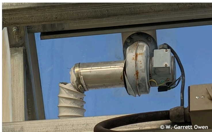
Figure 10. Vinyl drier vent hose was used, and UV light deteriorated the hose, thus inflating the double-poly with greenhouse air resulting in condensation. Photo by: W. Garrett Owen, OSU.
